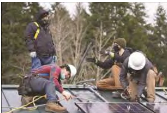
Volunteer installers show Quinault volunteers how to install the panels and conduit. Photo from Twende Solar
