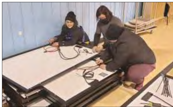
Sue Kalama works with volunteer installers to prepare panels for installation. Photo by Kelsey Moldenke
