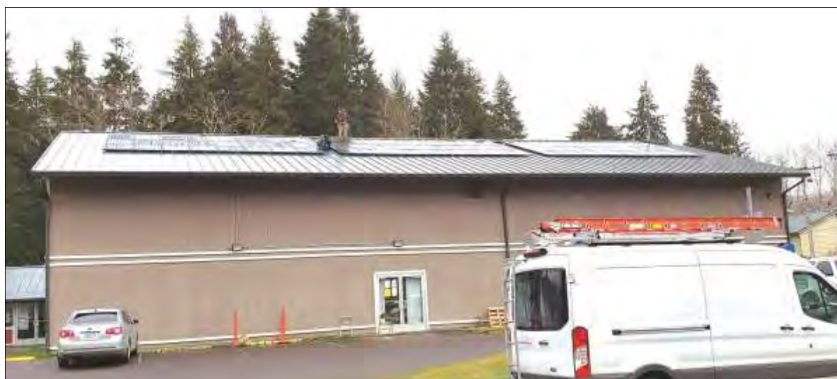
Full installed system on the Queets Community Center roof. Photo by Kelsey Moldenke
